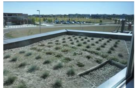
Newly planted green roof at Terwillegar Recreation Centre showing perimeter drainage, Edmonton, AB
