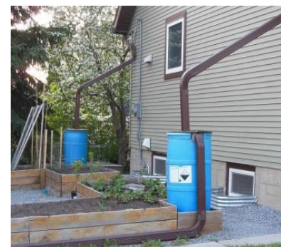
Residential rain barrel to harvest roof runoff for irrigating plant, Edmonton, AB.
